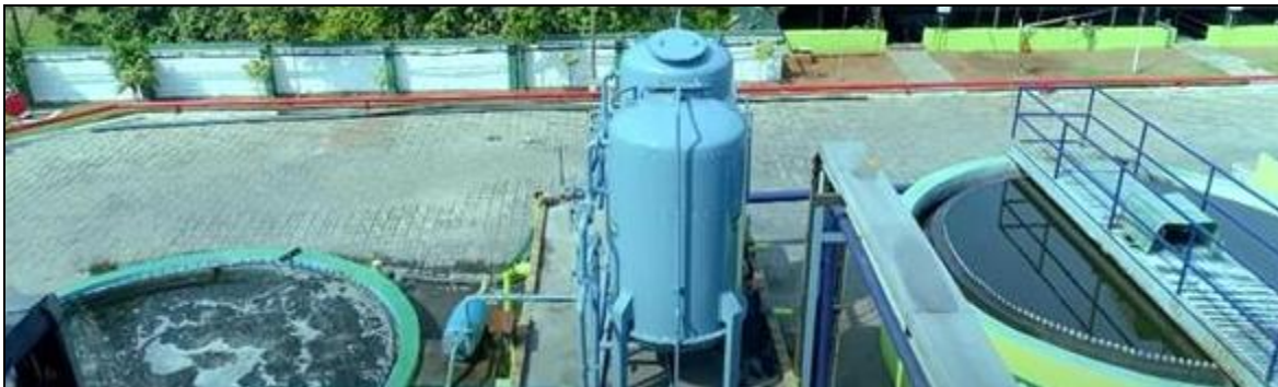
FIG. 7: EFFLUENT TREATMENT PLANT 9
